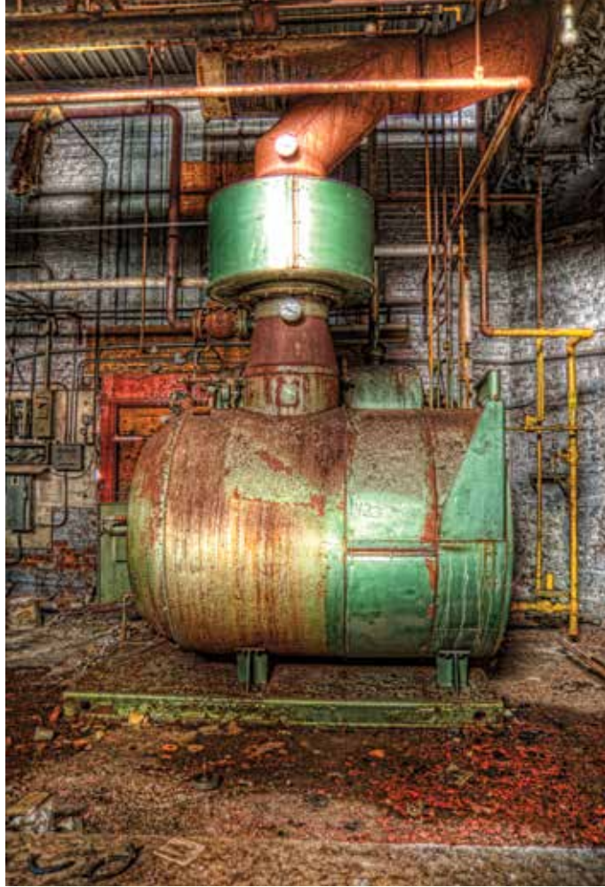
▲ “RUSTING AWAY” This was also taken at the Harvey Woods Factory. This old furnace was in the basement, and I loved the colours in the rust. I enhanced the vibrancy to help strengthen the rust effect in the photo and used some filters to help in the process.
